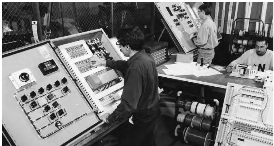
In-house assembly of control panel with PLC and operator interface terminal.
